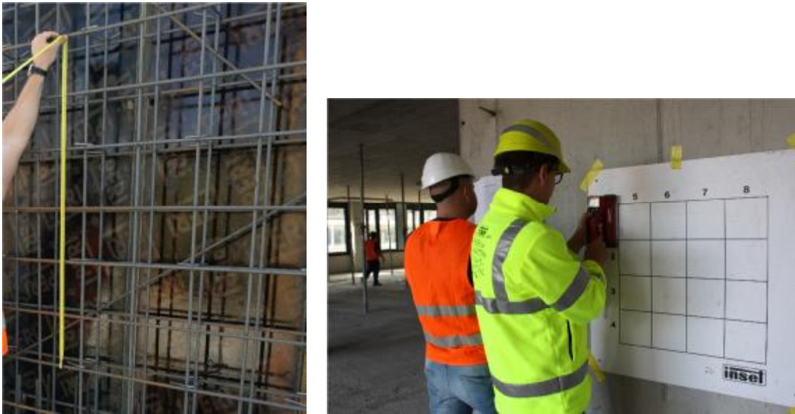
Fig. 2 To the left of the reinforcement before casting, to the right after casting
