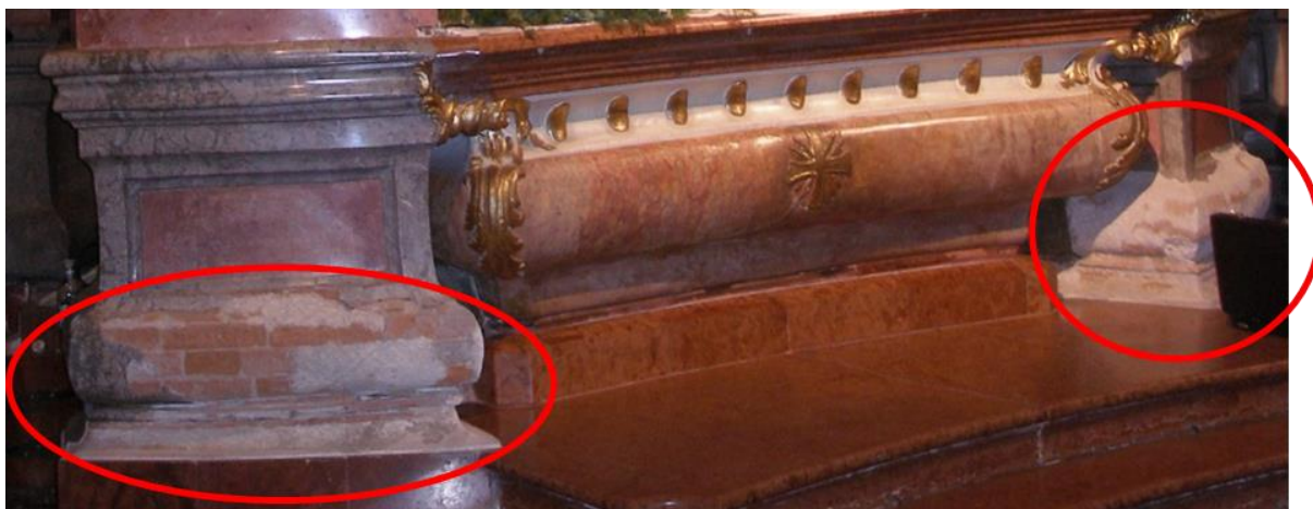
Fig. 6 Visible damages on the baroque altar.
