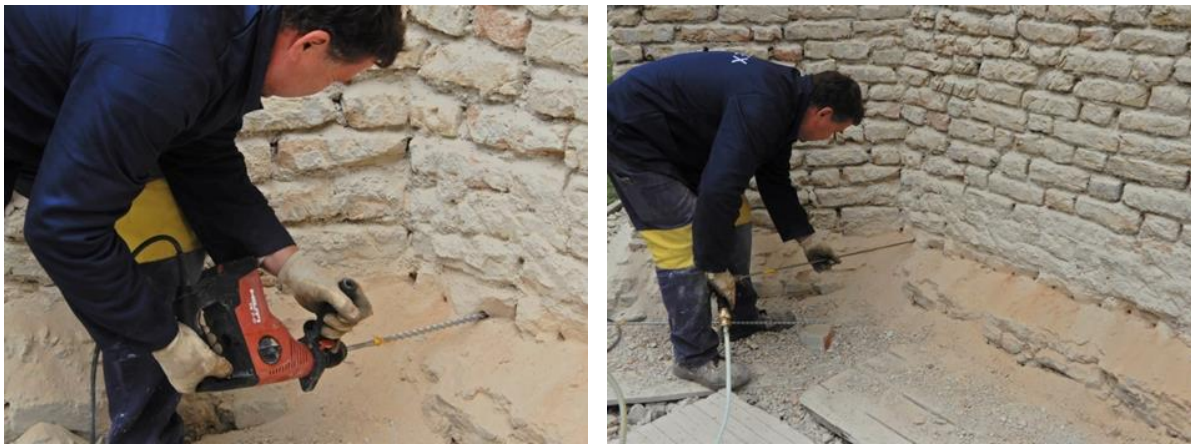
Fig. 5 Drilling boreholes (left) and injecting them with a creamy sealing barrier (right).
