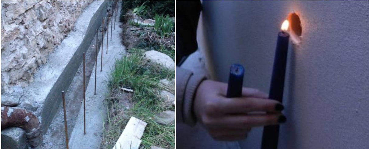
Fig. 3 The New made “ventilation” channel around the basements which stands, because of the use of concrete (left), beyond repair and the minimal air flow in this channel was proofed by a candle (right)
