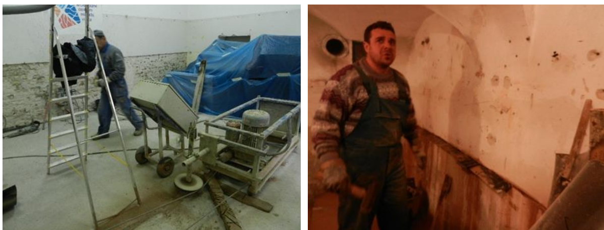
Fig. 7 Process of undercutting the masonry (left) and placing a solid insulation foil in the sawed gap (right).
