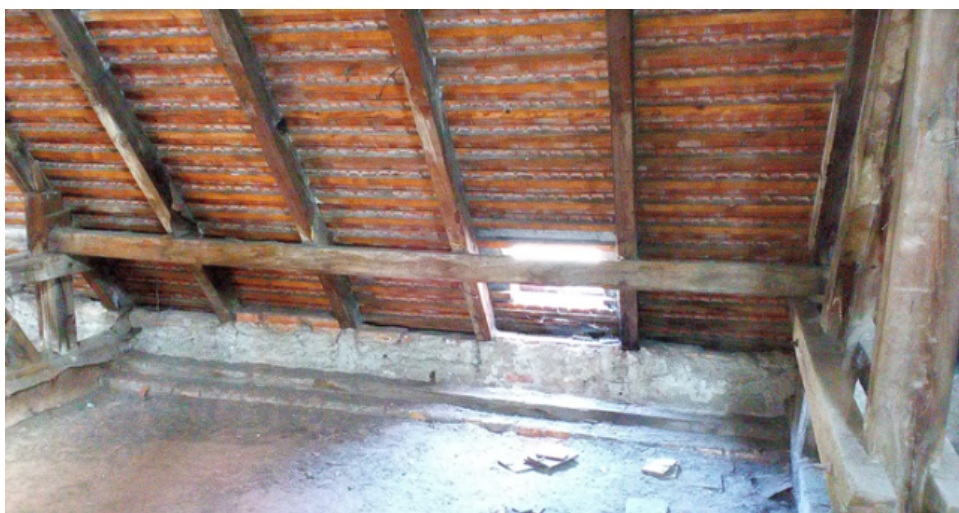
Fig. 7 Photo documentation of the damaged element (purlins)
